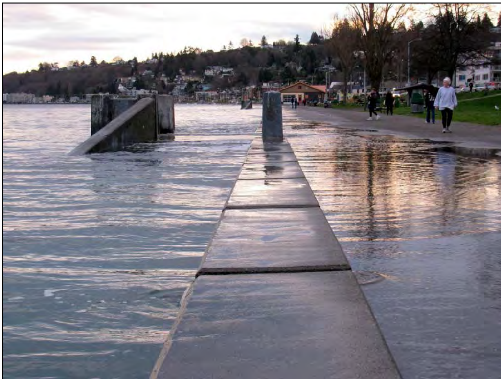
Figure A – 1: An unusually high tide in January 2010 caused water to spill over the seawall at Alki Beach in Seattle. Even modestly higher sea levels will cause the frequency of events such as this to increase, along with the potential for associated damage. (Photo by Hugh Shipman.)
